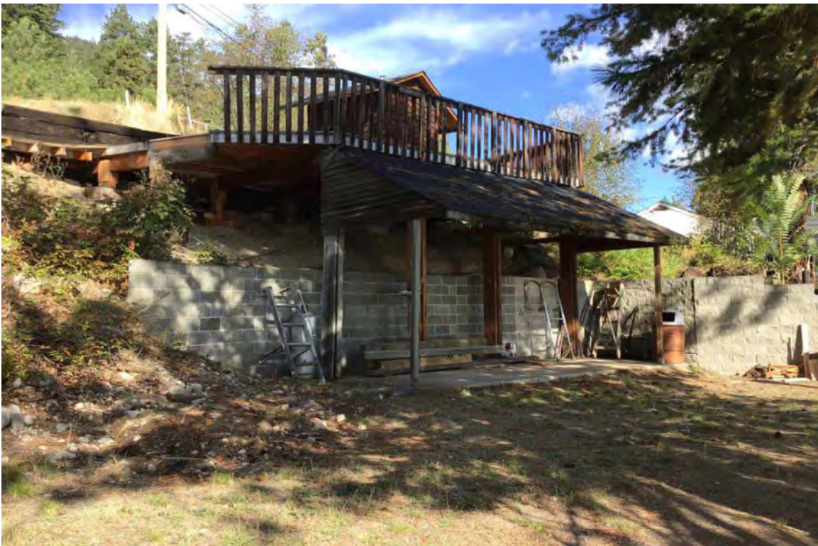
Photo 2. View looking northwest of the existing deck proposed for removal within the subject property.
