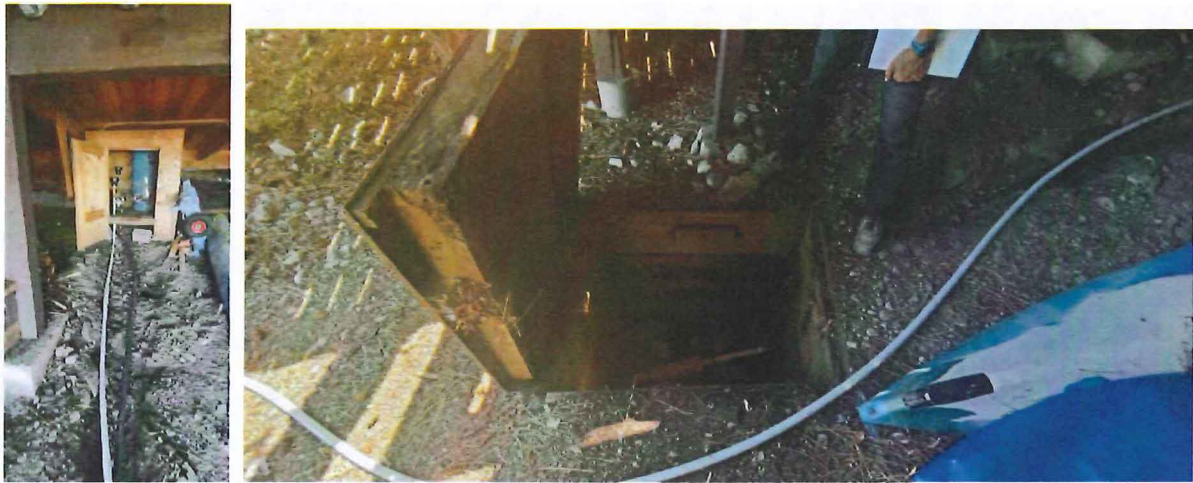
Photo 5 – Under cabin, buried water intake suction pump and control valve
