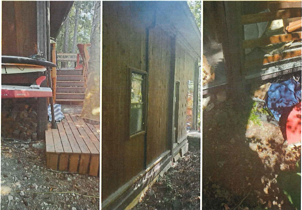
Photo 4 – Looking at – entrance to upper deck area, and south roof and downspout
