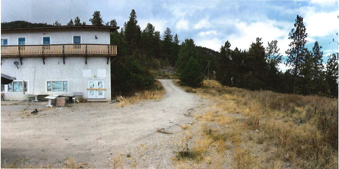
Photo 1: Looking northeast across the area of uncontrolled fill with the decommissioned building shown at the left. (Date of Photo – September 19, 2017).
