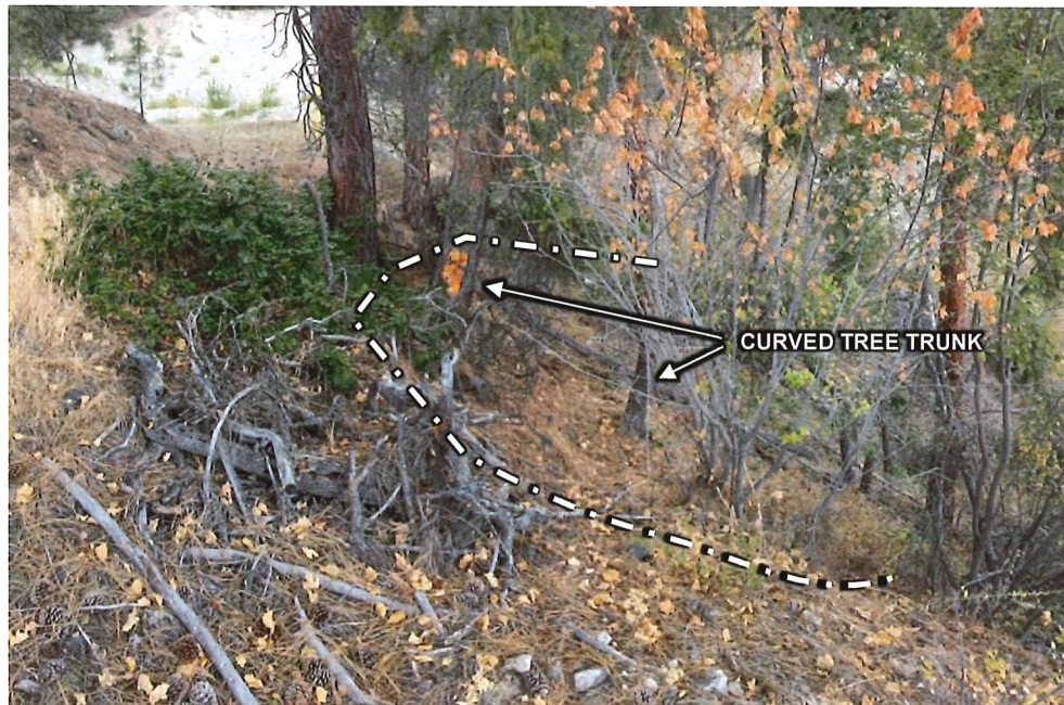
Photo 6: Looking west toward landslide 1 area. The concave area where historical movement may have occurred is indicated along with curved tree trunks that often indicate slope movement. (Date of Photo – September 19, 2017).
