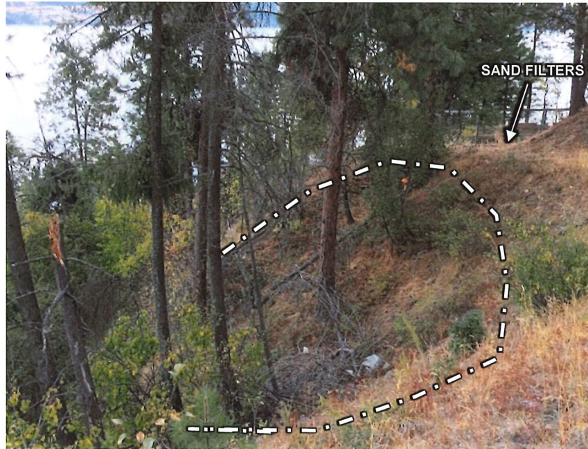
Photo 5: Looking east from Westside Road at landslide 1 area. The concave area where historical movement may have occurred is indicated. (Date of Photo – September 19, 2017).
