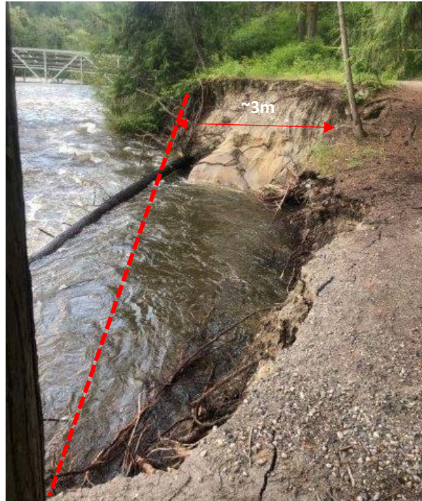
Photo 3 – Section of eroded bank near abutment showing 3m loss of back
