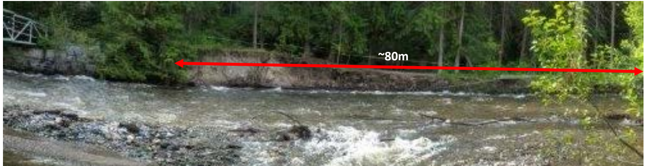
Photo 1 – Extent of 2020 erosion on right bank at Cedars Bridge
