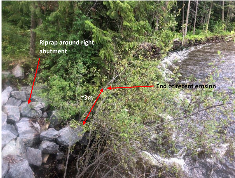
Photo 5 – Erosion ends ~3m upstream from riprap at right abutment
