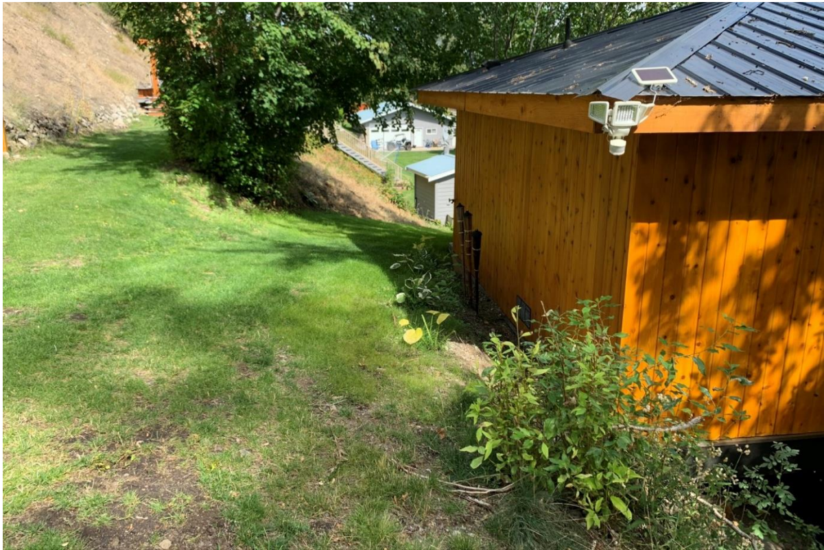
Photo 6. Photo taken from near the proposed new Sauna location. Only the back edge of the sauna building appears to be resting on the ground.
