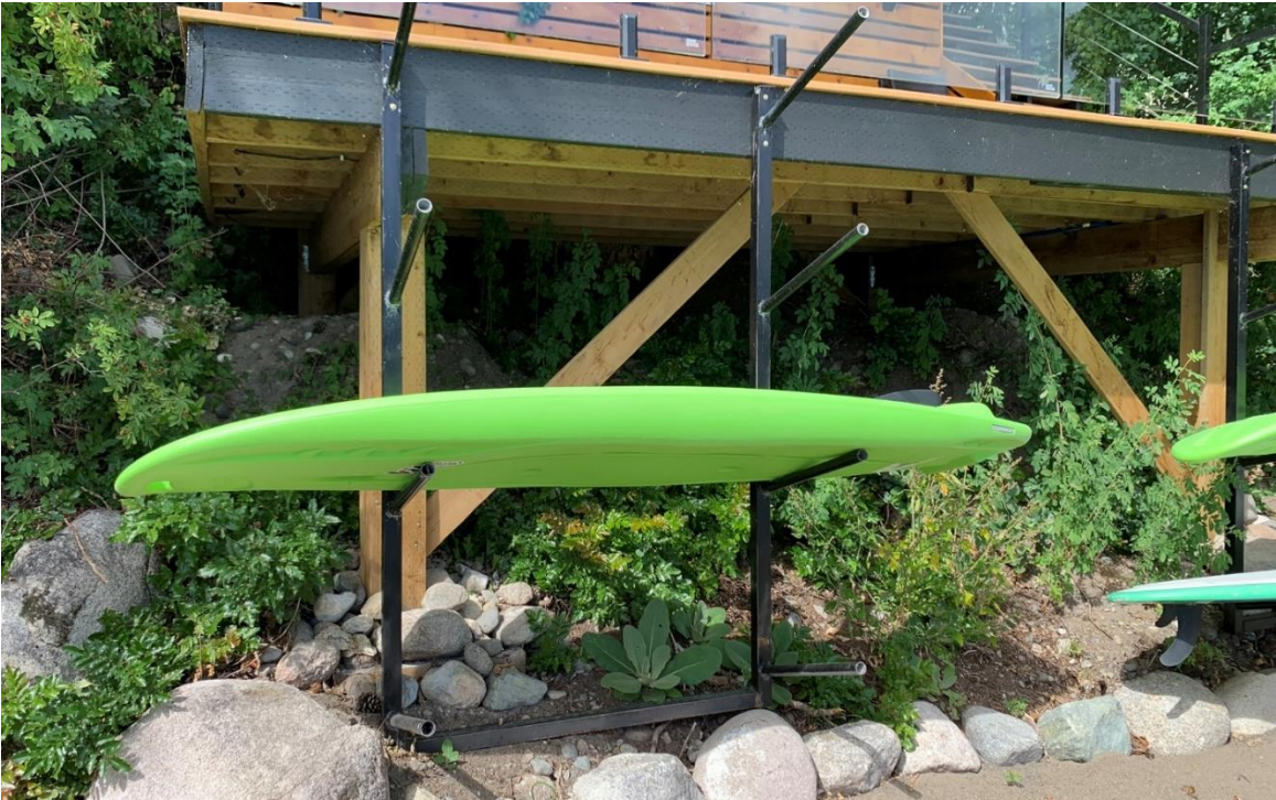
Photo 3. View of the underside of the Sauna building. Note native plant growth under it.
