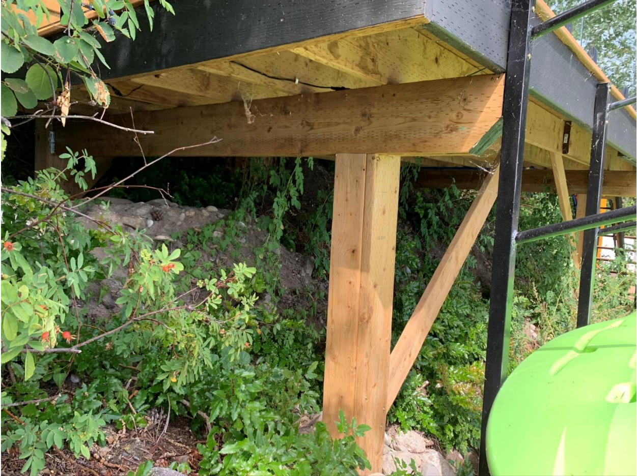
Photo 2. The front deck is supported by wooden beams on concrete blocks. These areas will be leveled and planted. There were native plants growing under the deck including Oregon grape, Nootka rose, snowberry, and woods rose. Each of these species spreads by runners and each is expected to proliferate once shade from the deck is removed.
