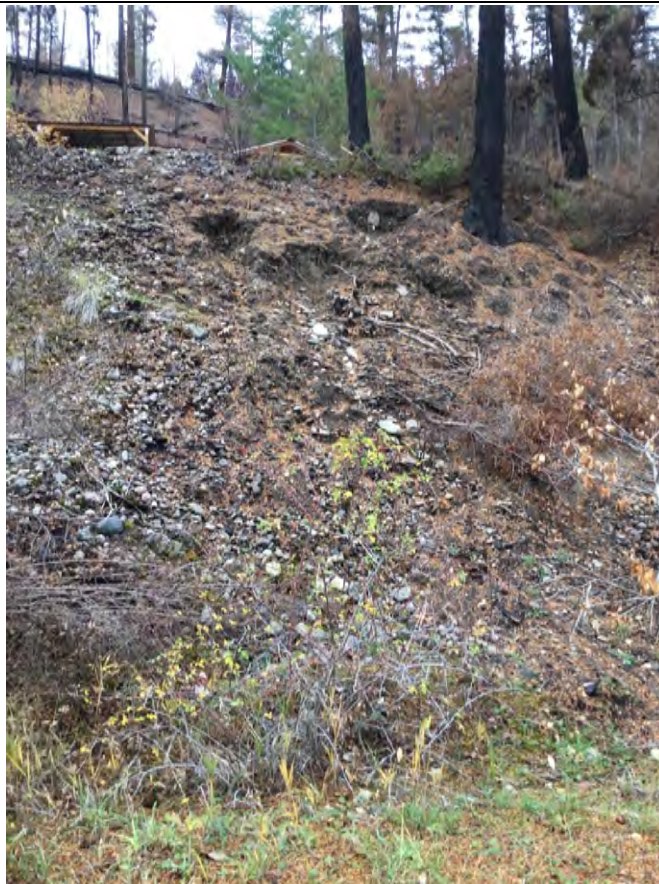
Photo 7: Shallow slope failures above upper Beachwood Rd (upper 43 Beachwood lot) (est. volume <10 cubic m)
