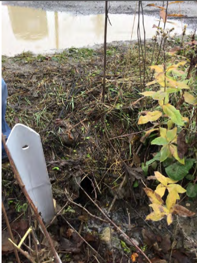
Photo 5: Culvert under Nerie Road, with flowing water from spring-fed stream (Buchanan Spring) and with contributing ditch flow.
