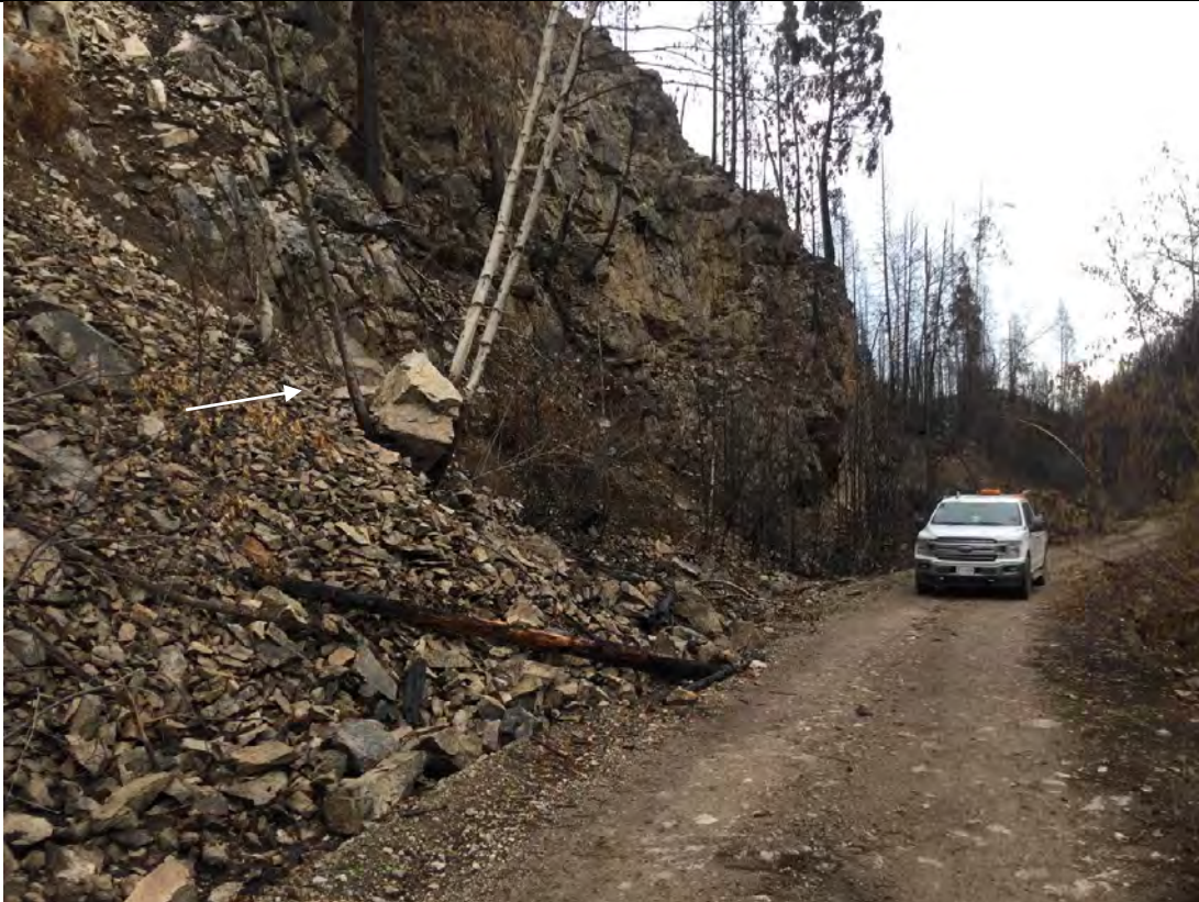
Photo 17: Example rockfall process along Whiteman Creek FSR
