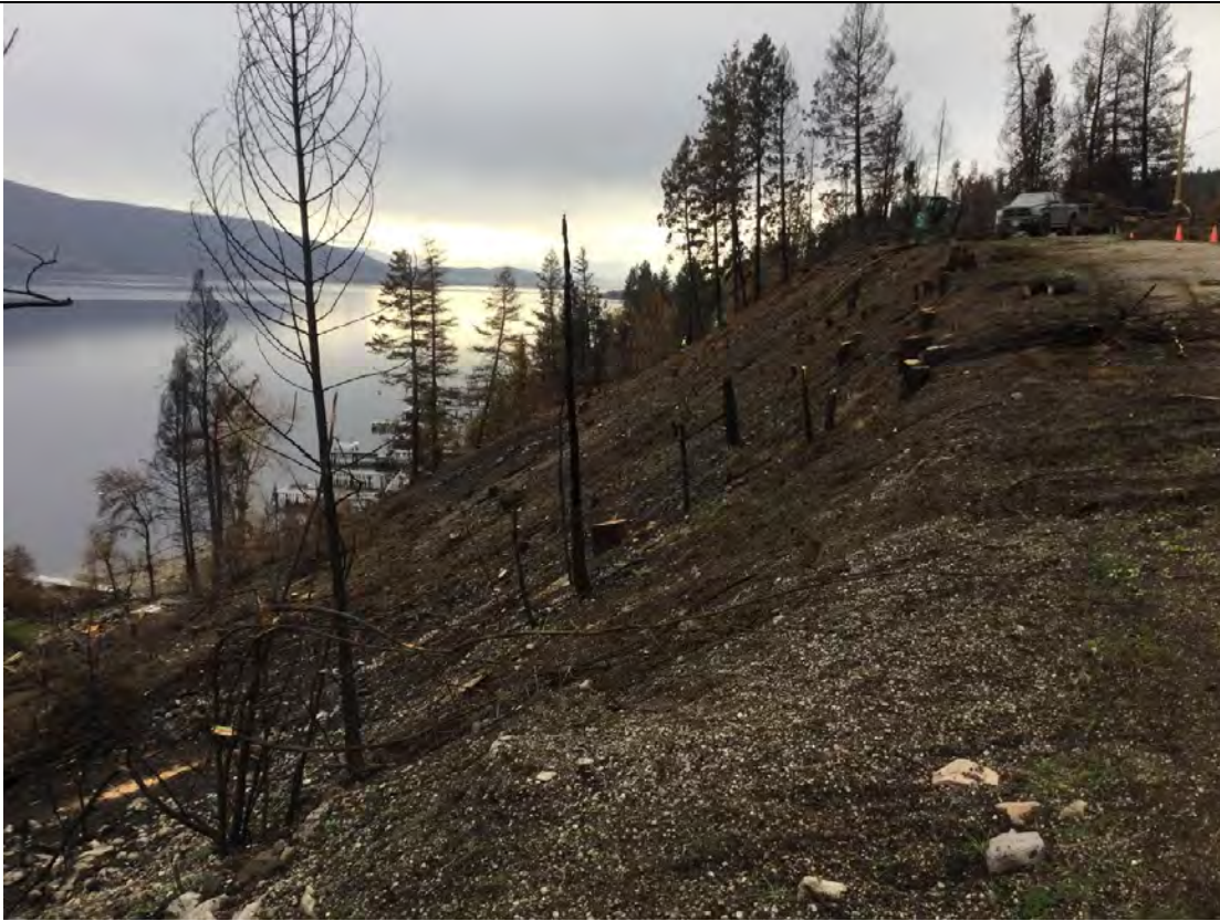
Photo 9: View across top of slope below upper Beachwood Rd. where burned trees were being removed.
