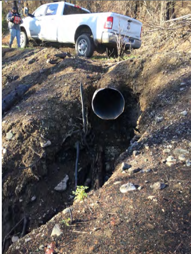
Photo 4: Failing culvert on Siwash Creek Road
