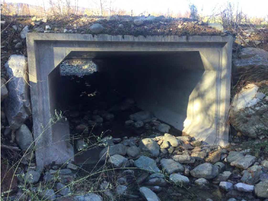
Photo 7: McGregor Creek concrete box culvert at Six Mile Creek Road crossing, ~250m upstream from Equesis Creek
