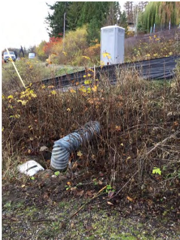
Photo 6: View of outlet of culvert under Nerie Road, Flow directed into a drain and buried culvert through lot (at 25 Nerie Rd)
