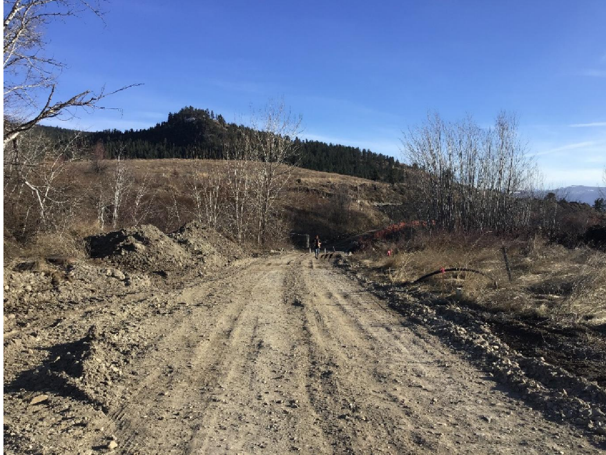
Photo 5. View of road associated with proposed upgrade to arch culvert at Sunset Ranch Drive over Rockface Creek, looking south.
