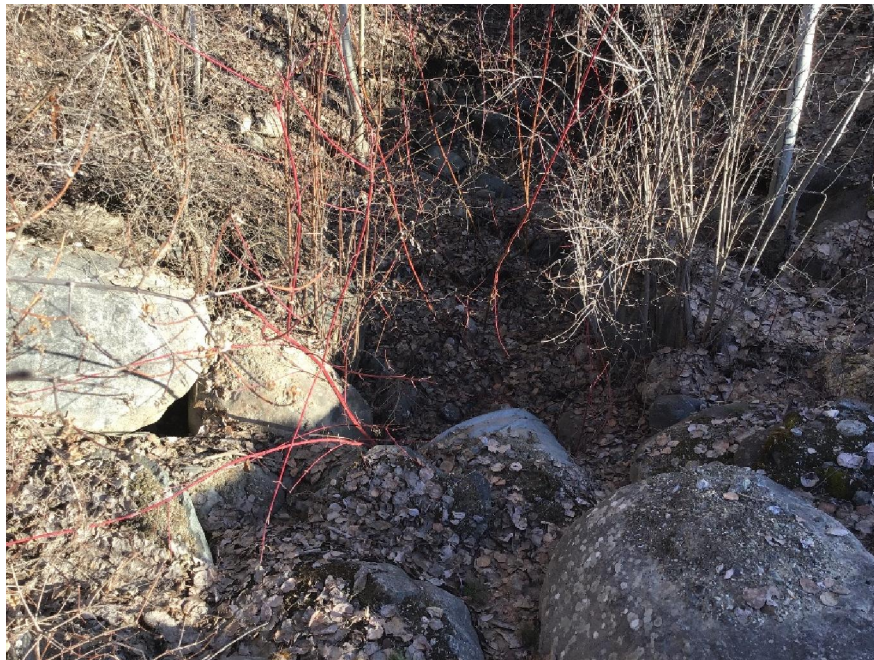
Photo 4. View of proposed upgrade to arch culvert at Sunset Ranch Drive over Rockface Creek.
