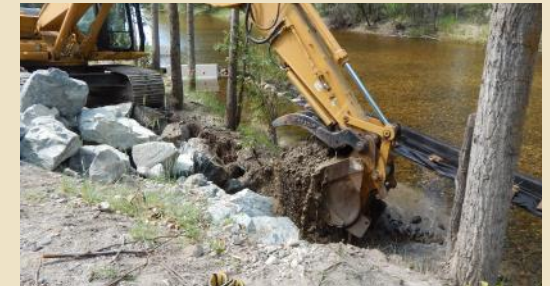
MCRI Phase 1 Habitat Restoration Project included dike setback construction (top photo) and channel restoration work (middle photo).
